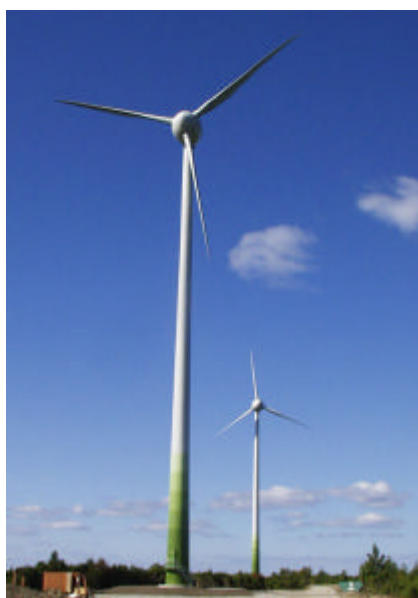
Figure 5 Virtsu Windpark, total capacity of 1800 kW (3x600 kW)
