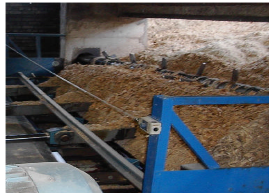
Wood chips feeding system - Broceni
