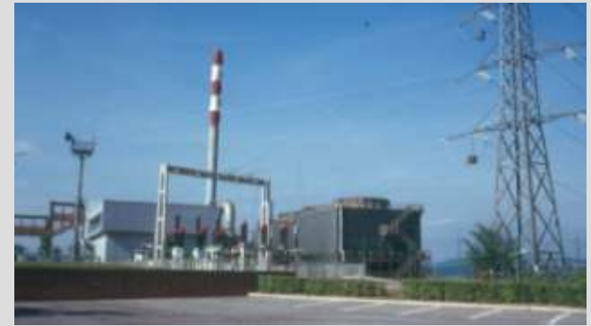
Power plant in Travale-Radicondoli, Italy
